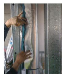
Continue lagging adjoining pipe area with the recommended overlap and joint treatment
